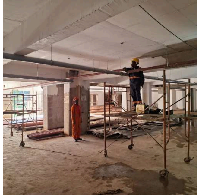
Basement Fire Fighting Piping
