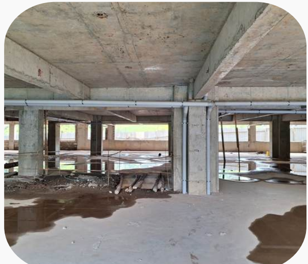
Basement parking plumbing
