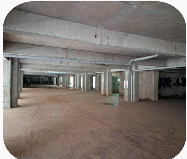
Basement parking plumbing
